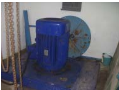
Pompes Station Sigoulette
