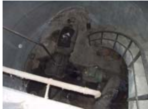
Station de pompage (pompes)
