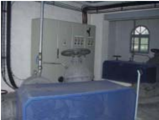
station Triquette refaite
