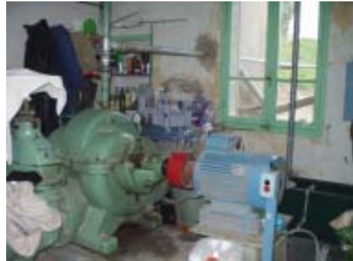
Pompe station Saliers
