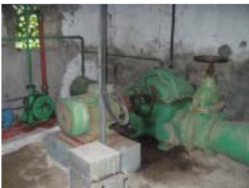
Pompe station Julian
