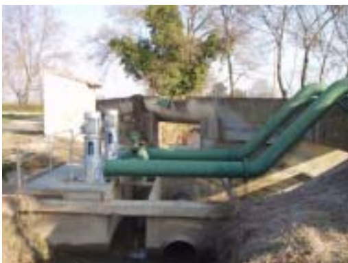
Station de Chalots - 2 pompes ALTA 350 l/s
